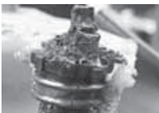
Figure 4 – Picture of a melted battery terminal
