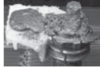
Figure 5 – Picture of a melted battery terminal
